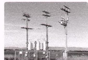
This is a voltage regulator site.
